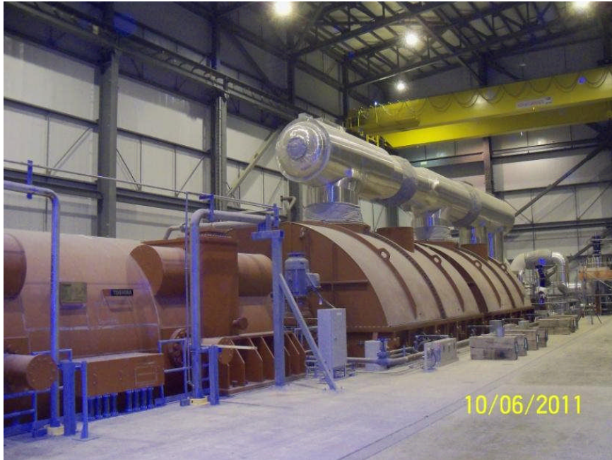
Unit 1 Turbine Generator Ready to Roll
