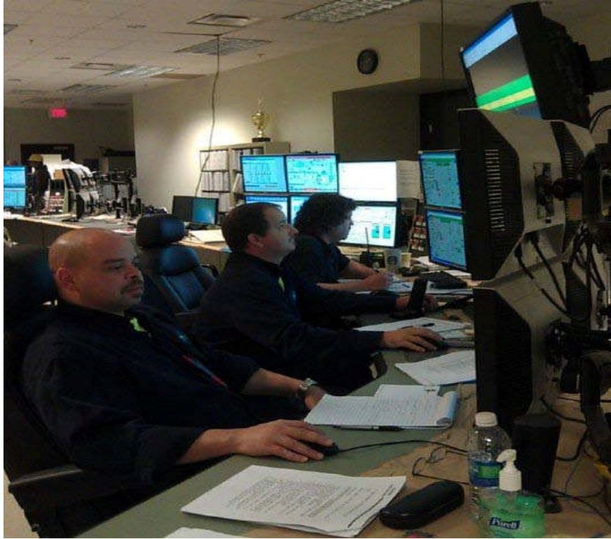
Unit 1 Control Room during Startup
